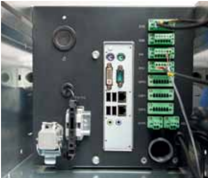
Rack cooling controller
