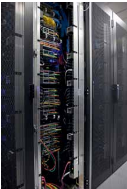
Knürr® DCM server rack for cooling with Knürr® DCL, Liebert® power distribution modules and integrated cable management.
