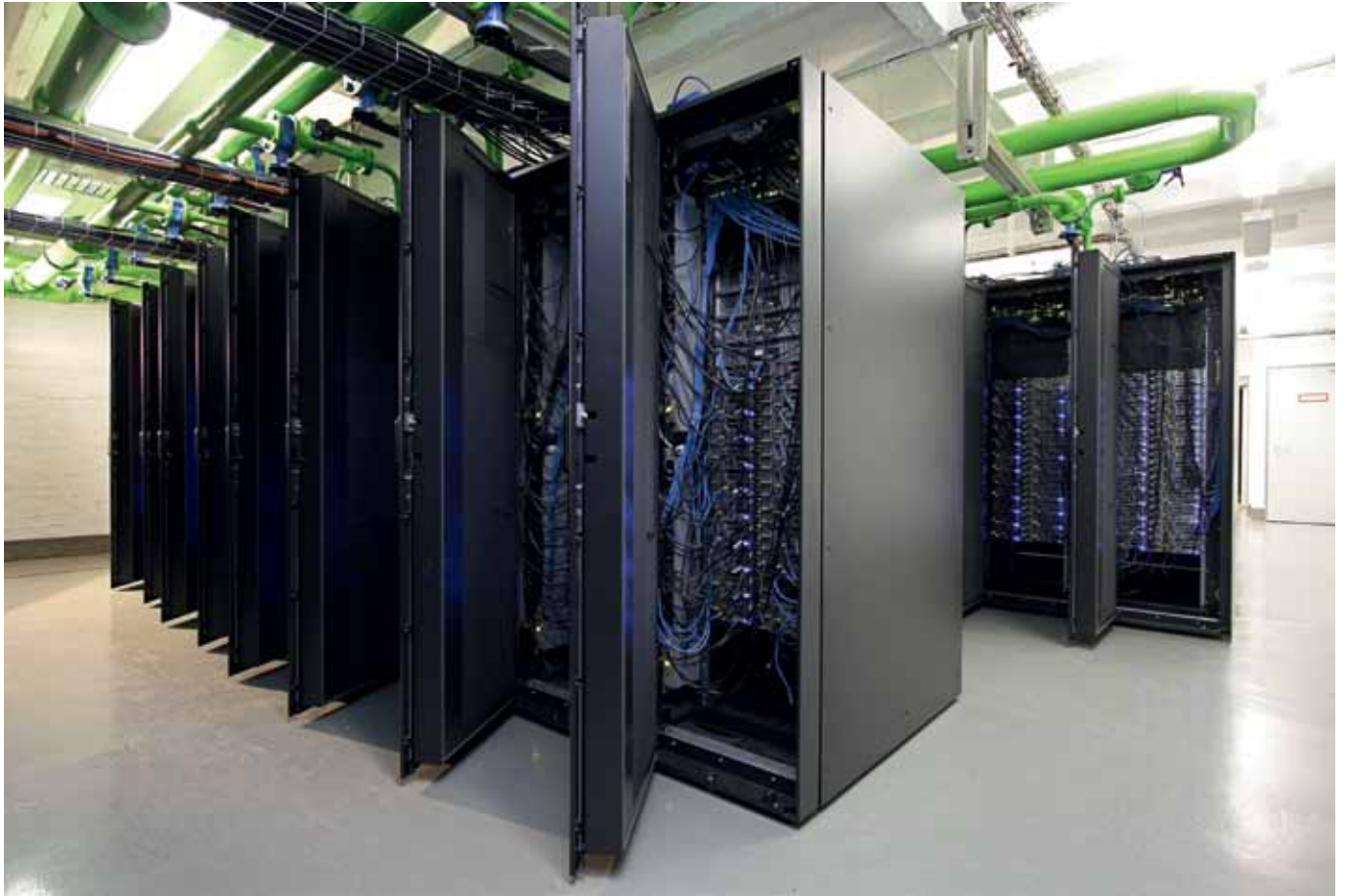
Knürr® DCD installation in Goethe University Frankfurt (Germany)
